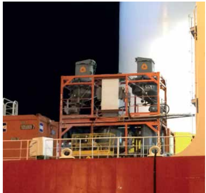
PHOTO: (Above) Core deployment of monopiles grouting from vessel (Below) Monopiles in situ
