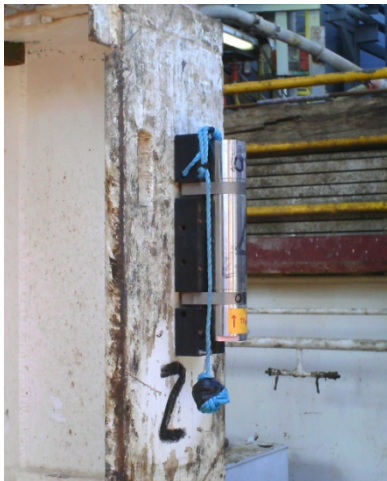
Data logger installed on BOP frame
